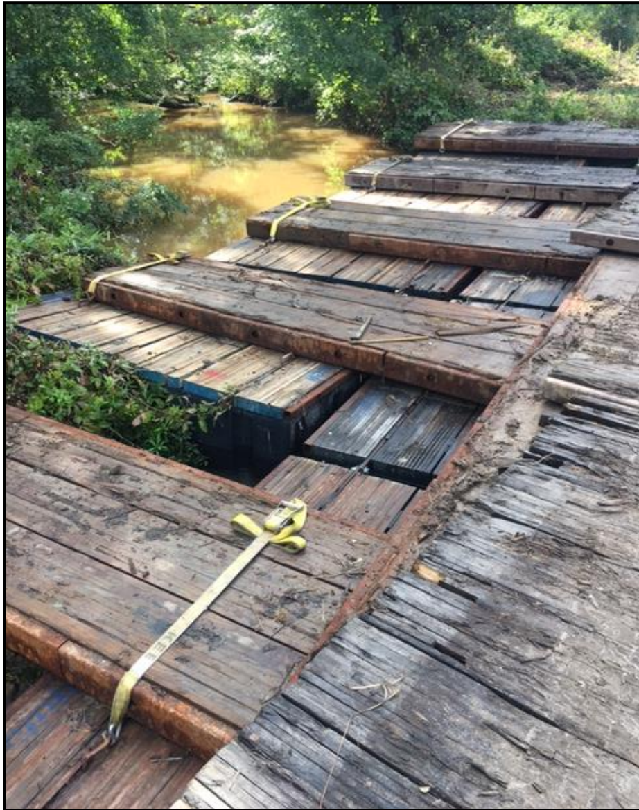
The mats use layering and buoyancy techniques to support the heavy construction equipment.
