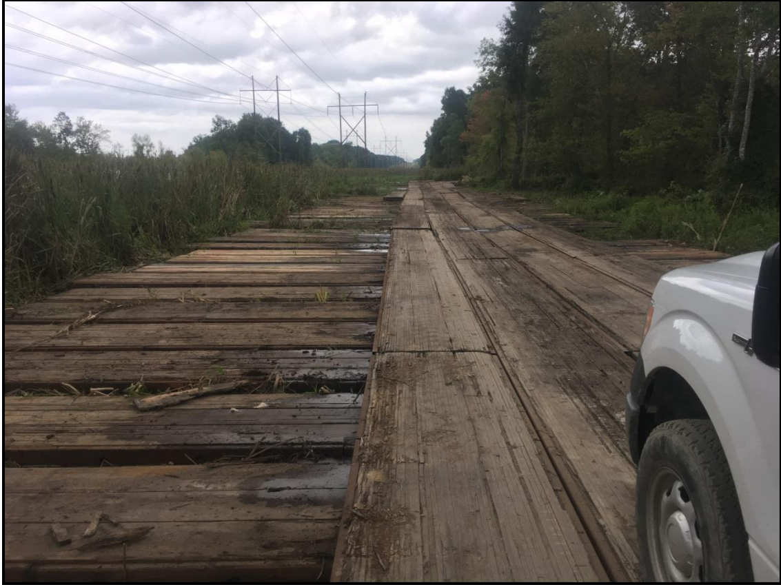
Emtek swamp mats on the eastern side of the 47 Line. These mats are rented, so a 'just in time' plan was put into place for their use.
