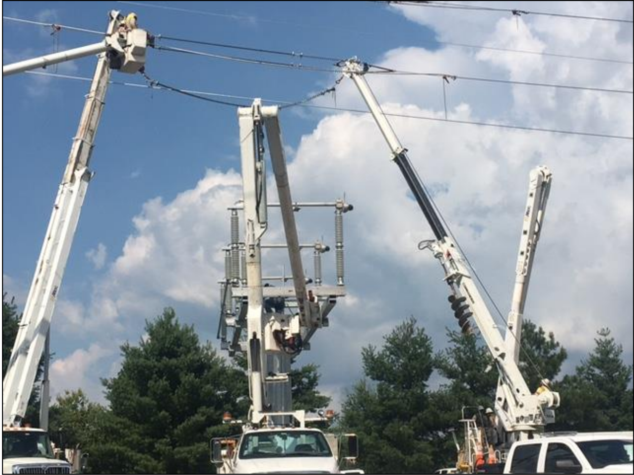
Installing floating dead end polymer insulators above new Switch 4729 at the Woodpecker DP Tap
