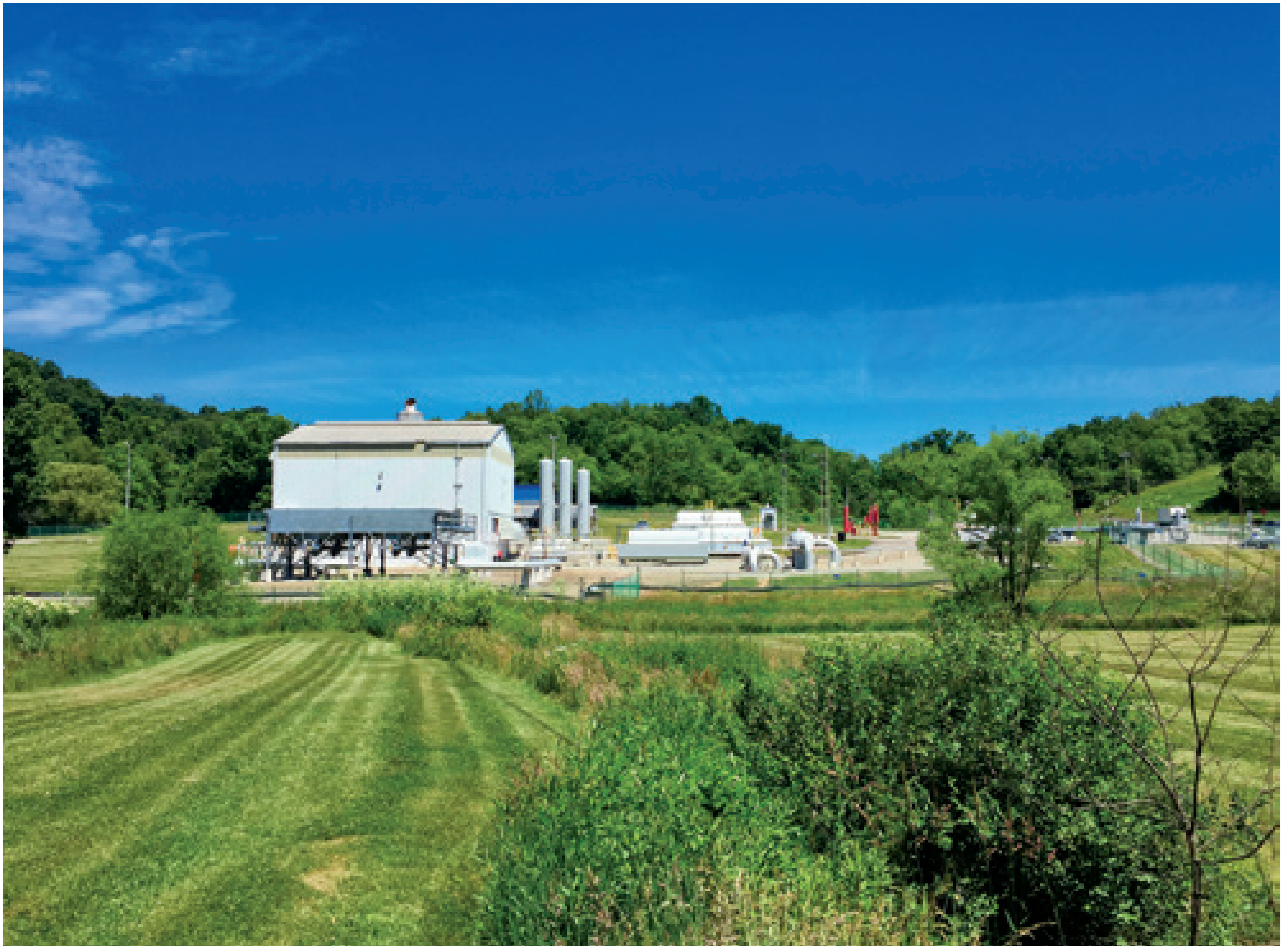
JB Tonkin Compressor Station Westmoreland County, Pa.
