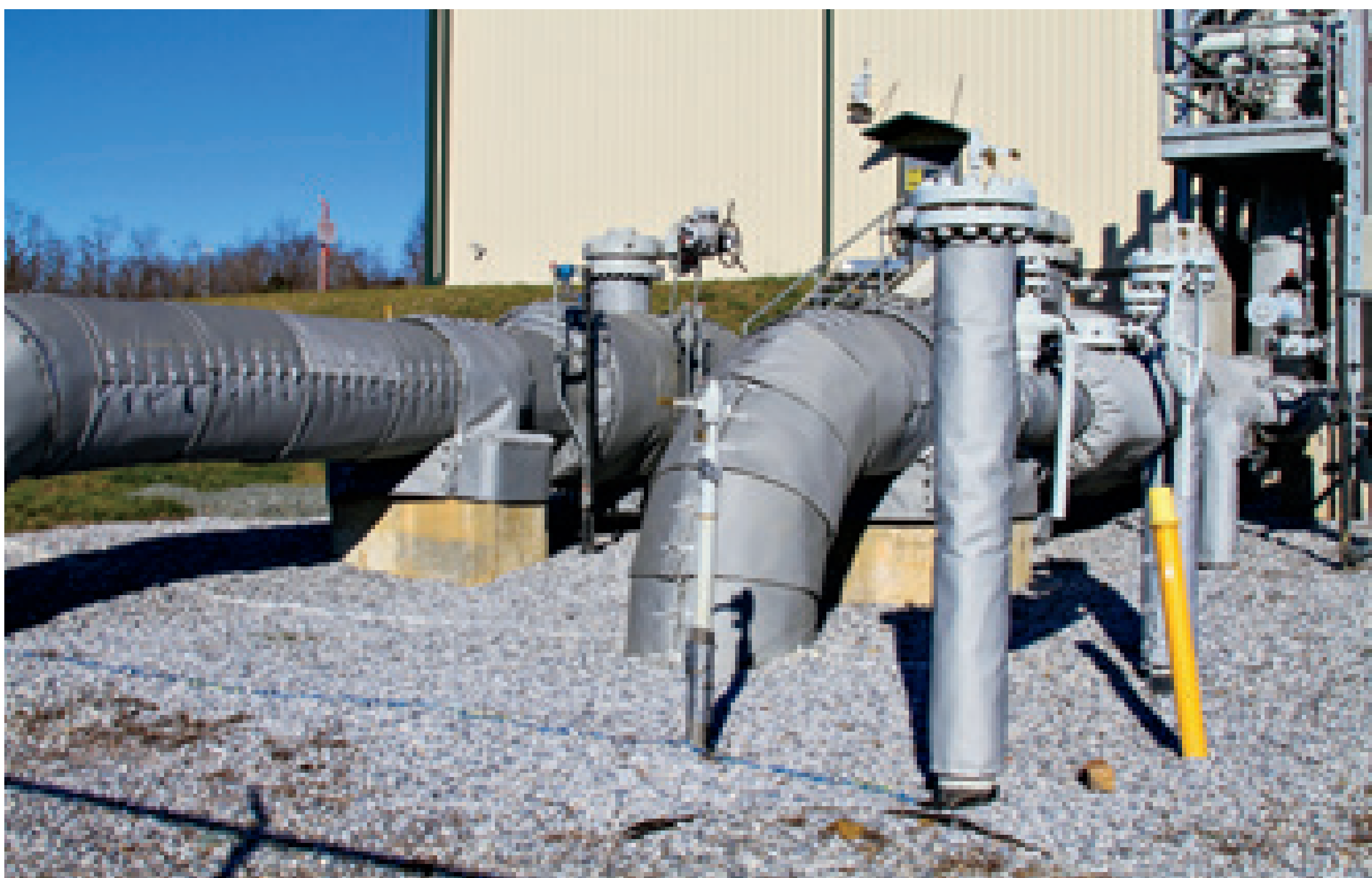
Acoustic insulation shown on exterior pipe sections
