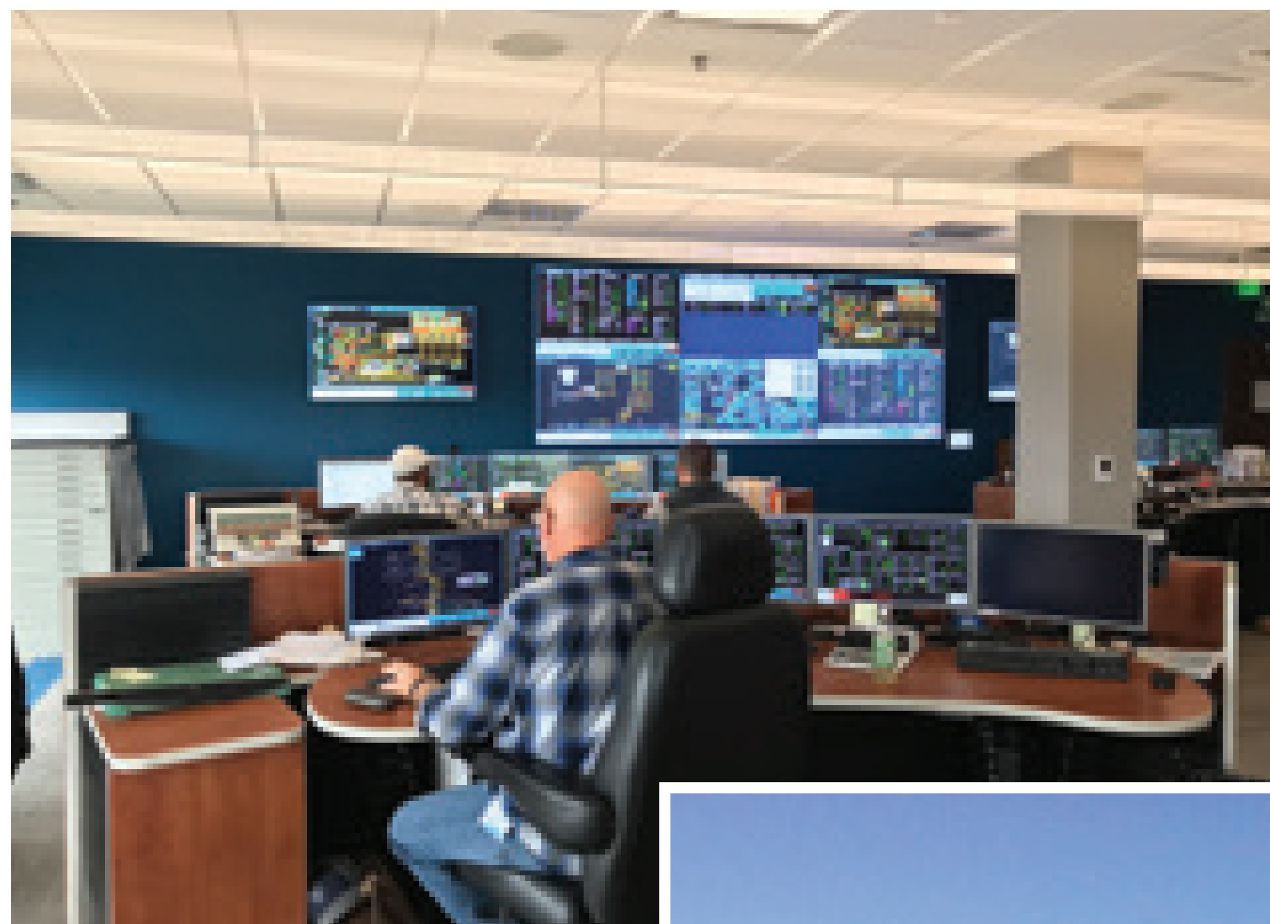
Dominion Energy's Gas Control Center operates 24 hours a day, 7 days a week.
