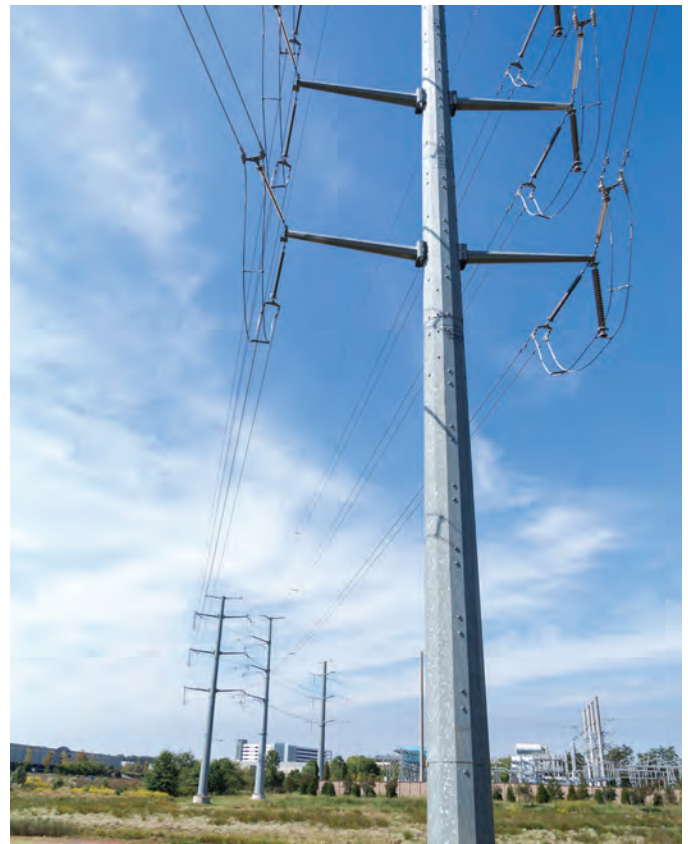
Transmission lines; Loudoun County, VA
