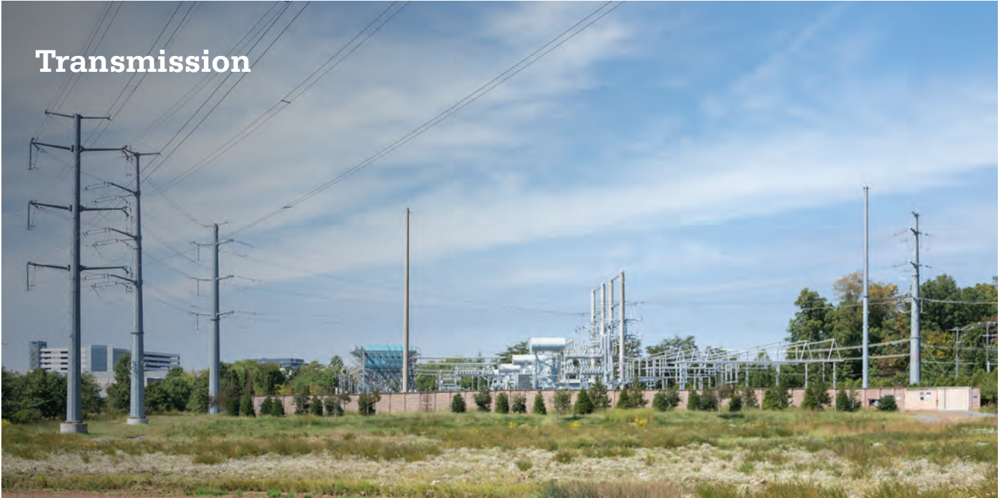
Transmission lines and substation; Loudoun County, VA
