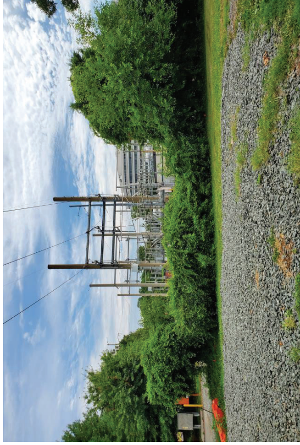
P2 - View north of existing transmission lines and Tysons Substation.
