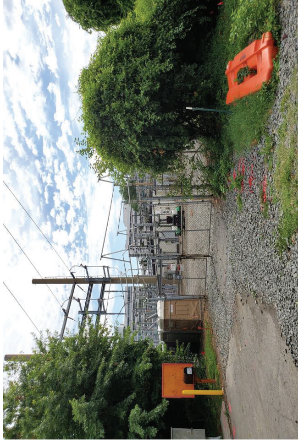
P1 – View north of gated southwest entrance to Tysons Substation.
