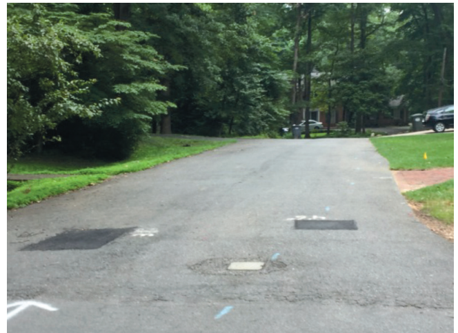
Roadway with potholes patched with asphalt.
